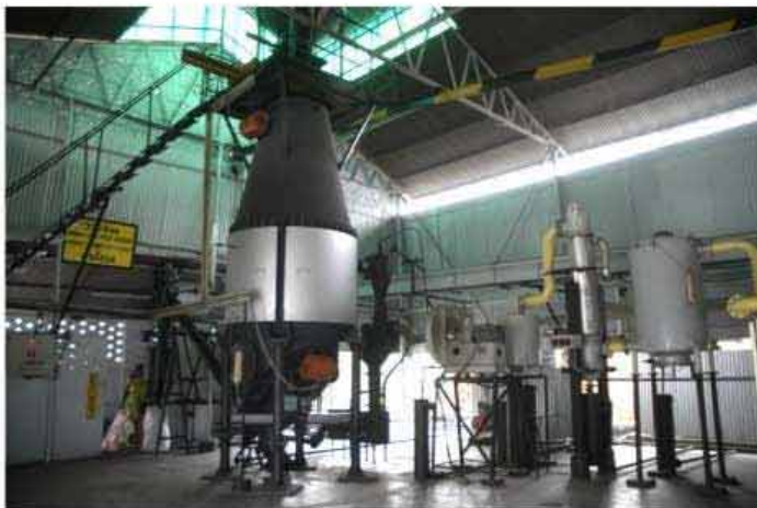
Rice Husk based 250 kWe Power Plant, India
