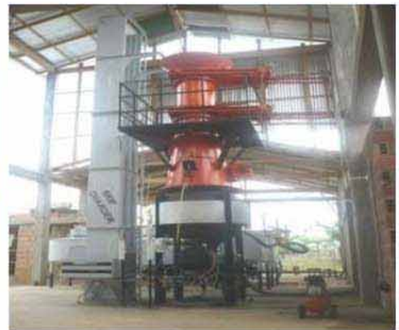
40 kWe Power Plant, Colombia
